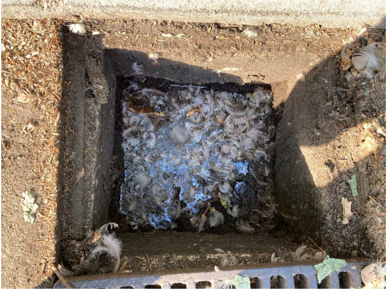
Photo 1: Drop inlet where the inspection was completed because of the outfall pipe being under water. Some standing water was observed, but no flow. Deep sediment in DI is blocking entire outfall pipe.
