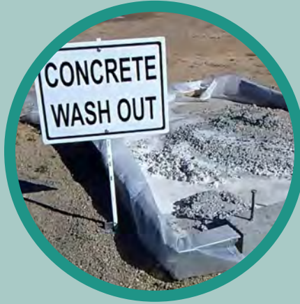
Construction Site Concrete Washout
