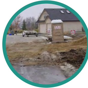
Poor Construction Site Practices
