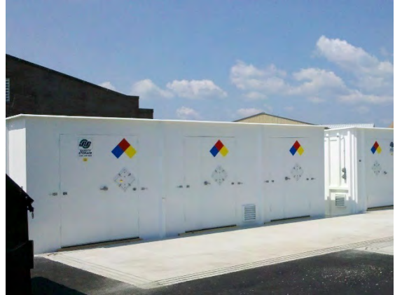
Figure 190. Outdoor storage of hazardous materials ( SafeSpace ).
